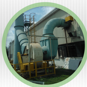
Welding Fume Extraction
