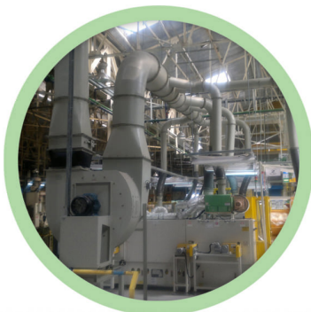
Fume Extraction System
